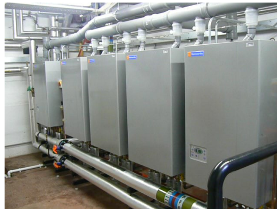
Truro Cathedral's New Boilers
